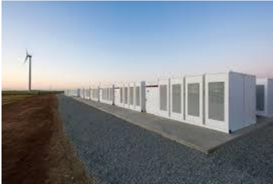
Tesla Battery in Australia
